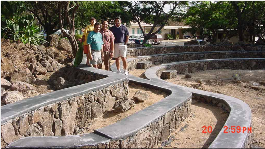
The Native Hawaiian Healing Center amphitheater is nearing completion. Stay tuned for further construction news.
